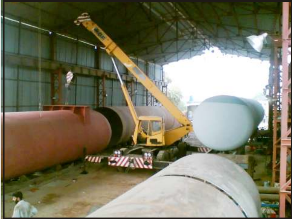
LPG STORAGE TANK
