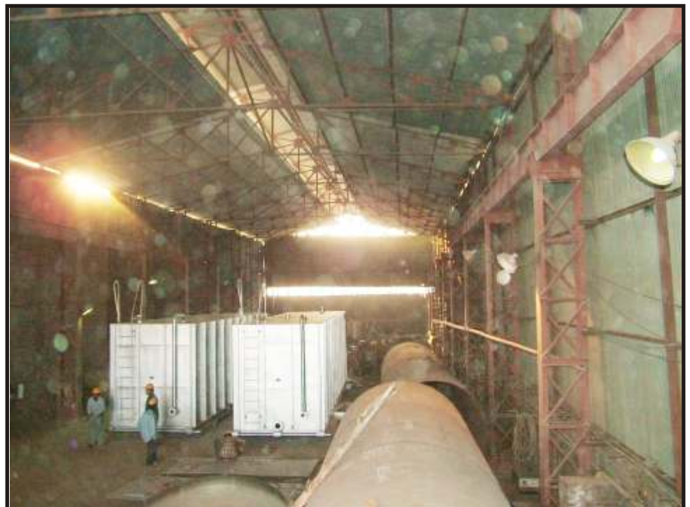
500 BBL CRUDE OIL TANK - OPII
